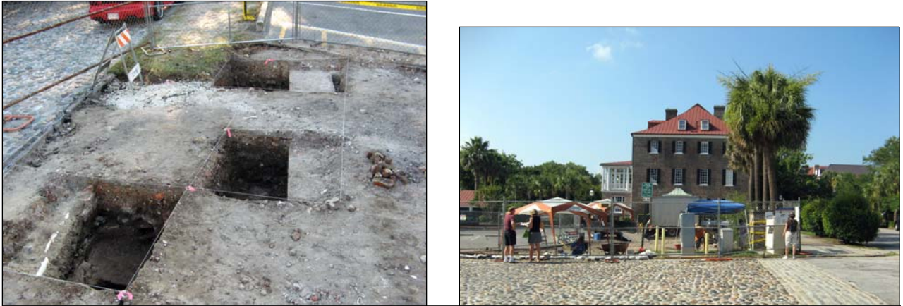
Figure 38: Initial excavation units expose Feature 9, foundation of the Vanderhorst north tenement; The extant Vanderhorst south tenement in background.
