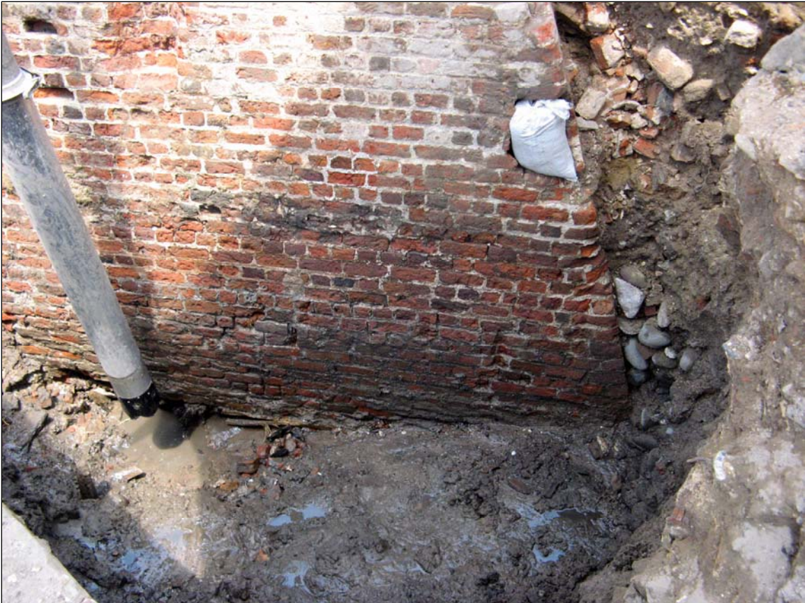
Figure 47: Excavations to the base of the brick redan, below water table, with aid of the vacuum truck.
